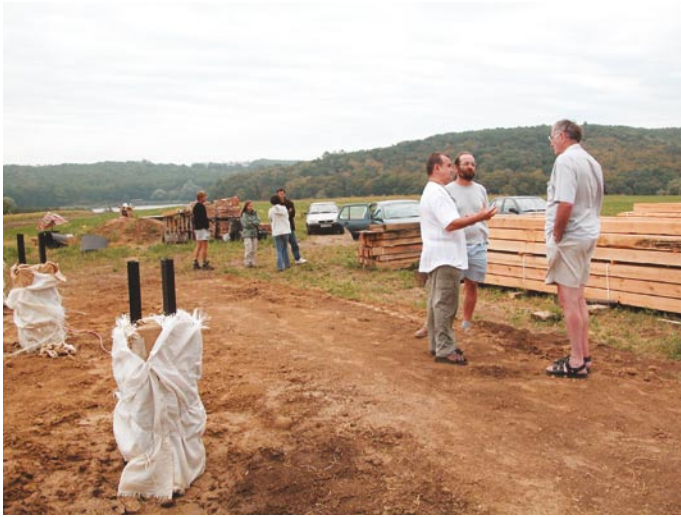
Top: Géza Varga, Imre Killian from Gyurufy and Ross Jackson at the ecovillage building site.
